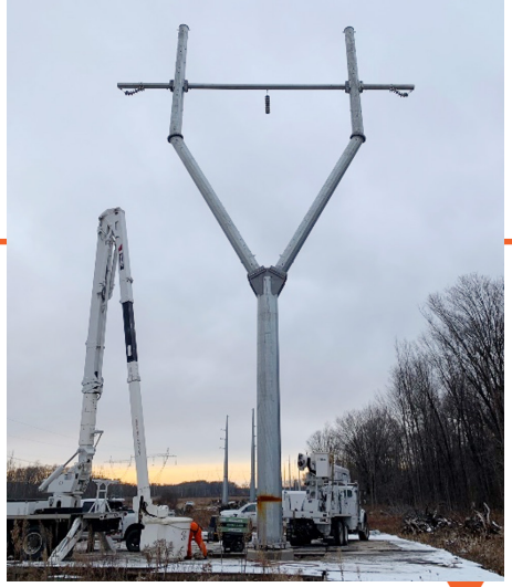
Y-type transmission poles.
